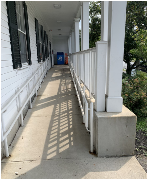
Entrance ramp hard to navigate with wheelchair; often blocked with strollers at bottom
